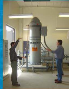
Calleguas MWD, Thousand Oaks, California ASR Well
