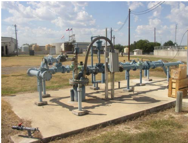
Figure 3-4: ASR Well R-1 at Kerrville Water Treatment Plant
